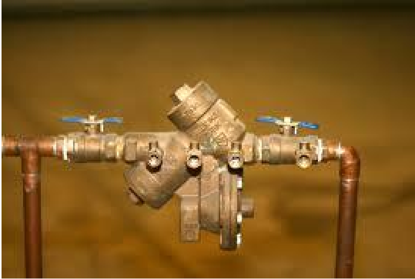
Irrigation System RPZ
