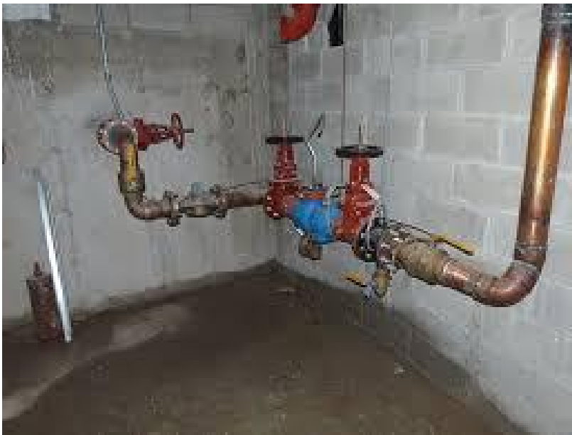
Fire Suppression System RPZ
